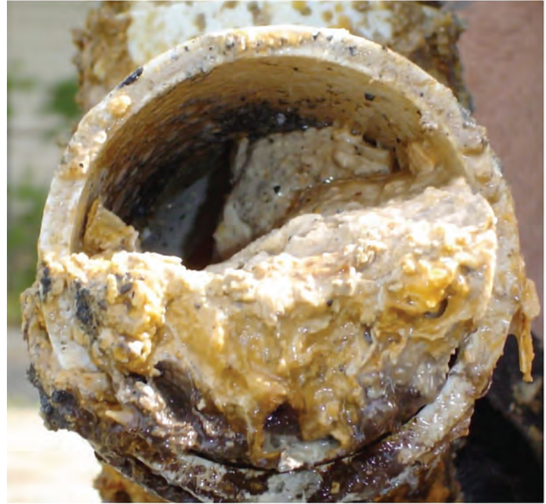
Gross fatbergs grow and block our sewers. Photo courtesy of Portland Bureau of Environmental Services.
