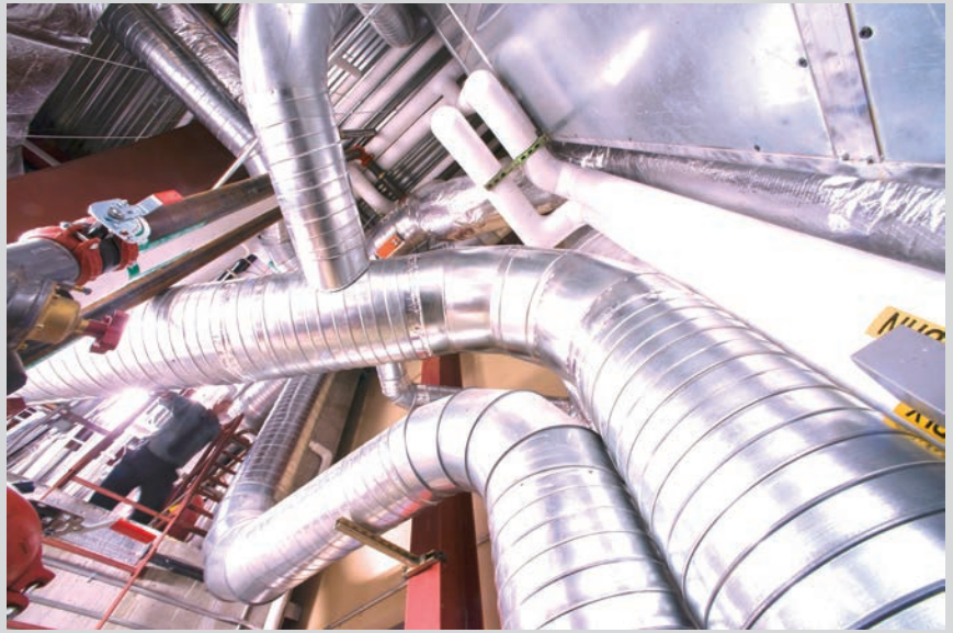
Industrial Art - metal clad gas flues soar up a main shaft.
