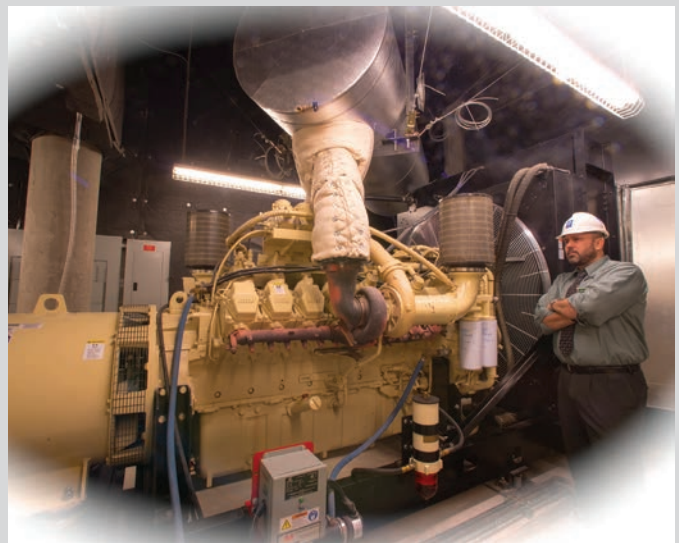
Keeping Lights On - facility boss John Hart with 1,000 kw diesel generator which provides backup emergency power.
