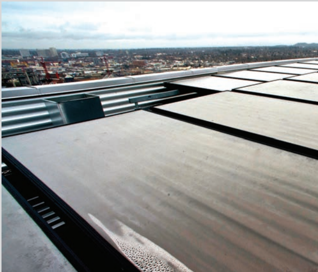
Rooftop Recovery - These solar panels, at the very top of the building pre-heat domestic hot water. The area is known as floor 31-1/2.
