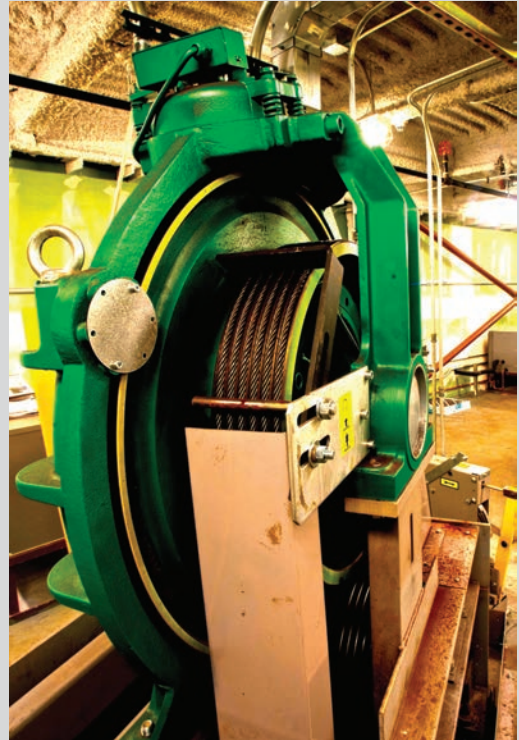
Getting a Rise - Incredibly strong cables run four Tower building elevators and two Terrace elevators. Tower elevators are powered above the 30th floor.
