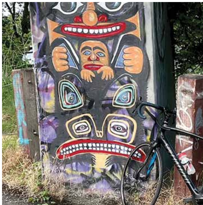
Grffiti on a column supporting the Ross Island Bridge.
